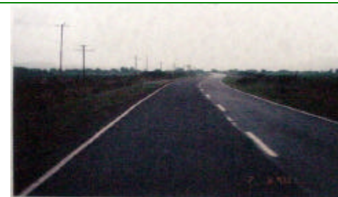
Construction of 5 km of Paved Road from San Jerónimo to Abrego US$2,829,454
