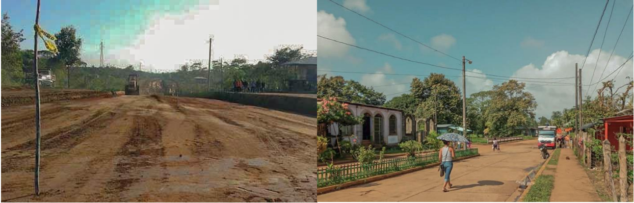
Figure 1 Streets of Kukra Hill (Before and after)
