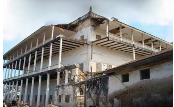
Figure 2: A corner section of the House of Wonders that collapsed in November 2012 (Source: WMF 2017)
